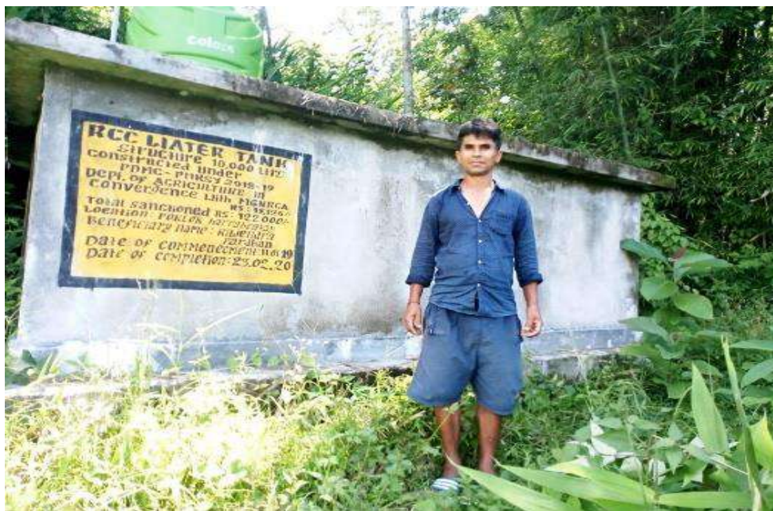
10,000 LTRS RCC WATER TANK NAME OF LAND DONOR: AJAY CHETTRI LOCATION: SAMATAR
